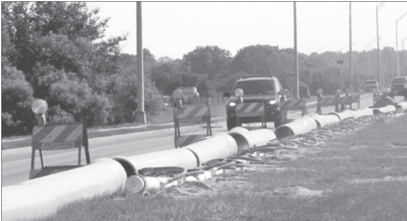
The County is struggling to keep pace financially with the demands of road construction and road improvements east of the interstate I-75. Lakewood Ranch Boulevard is the site of construction as workers install sewage mains.
